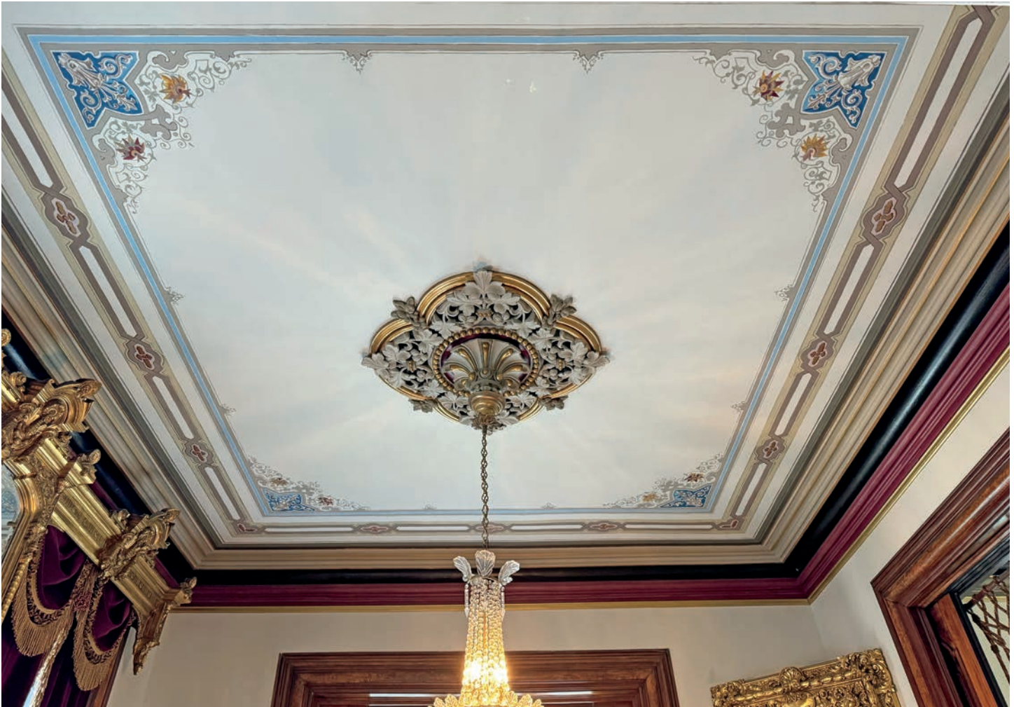
The first floor dining room ceiling after being restored and repainted Photo courtesy of Joy Christensen
